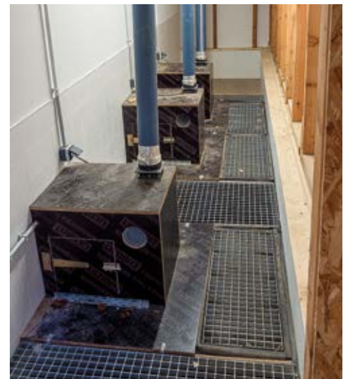
Solids management system.
