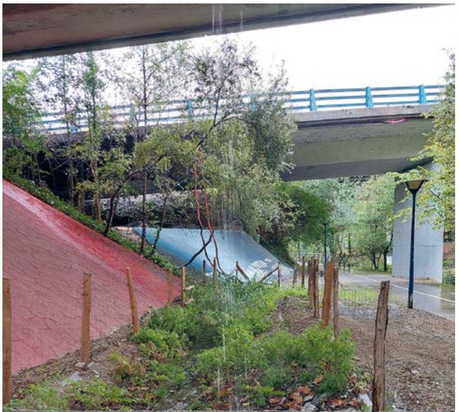
Runoff from the motorway viaduct is sent to the naturalised ditch below.
