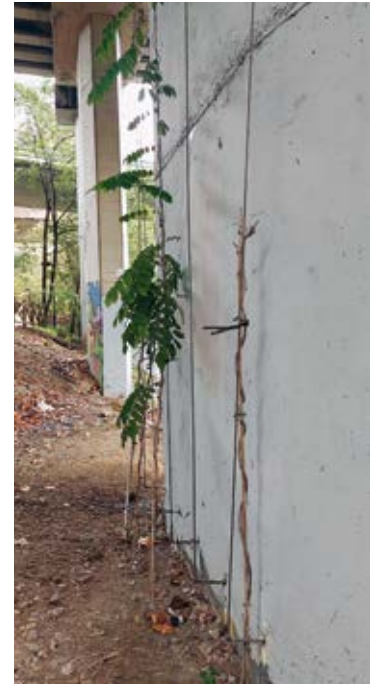
Cables anchored to the pillars, providing separation.
