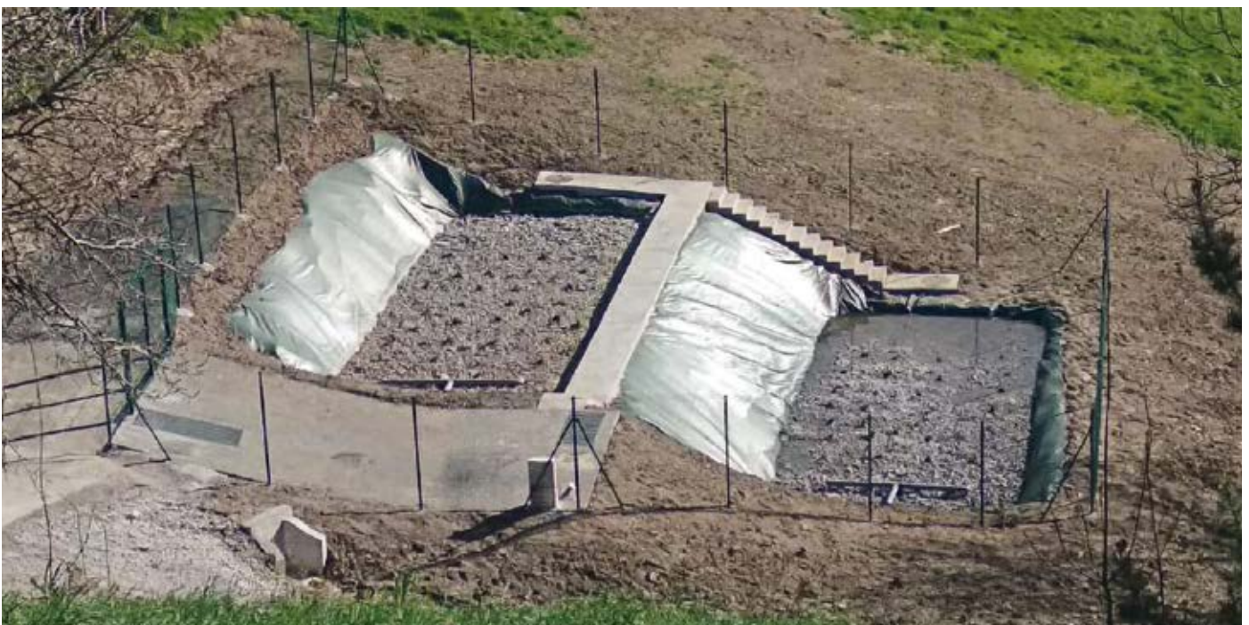
General view of the artificial sub-surface horizontal flow wetland using macrophytes in the Merru district.
