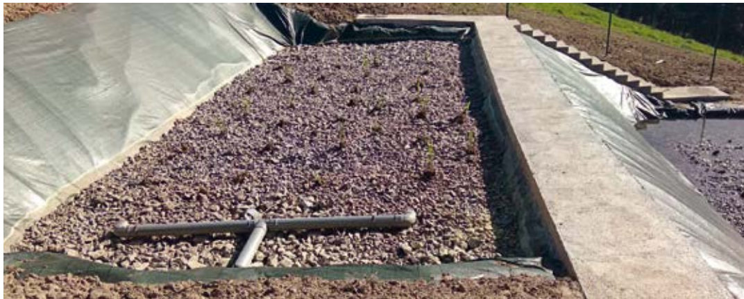
Lower basin of the constructed wetland, showing the gravel filtering substrate with different grain sizes and a thickness of 60 cm, in which the aquatic vegetation is planted.
