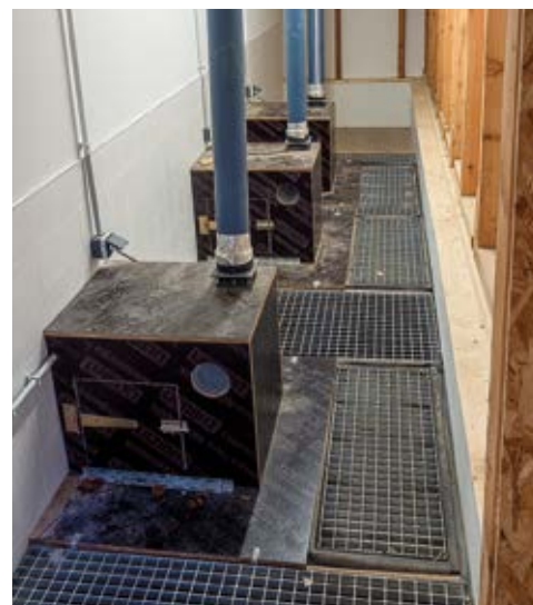
Solids management system.
