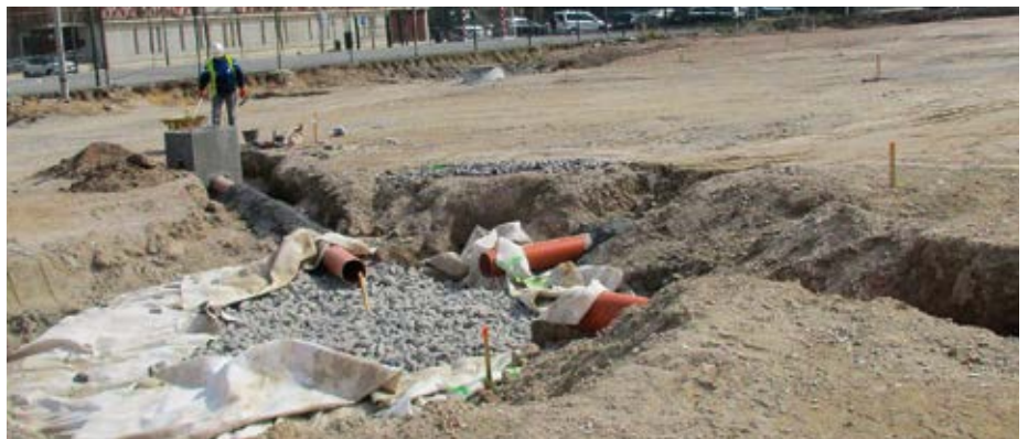
Rainwater channelling system using HDPE pipes that discharge into the gravel column.
