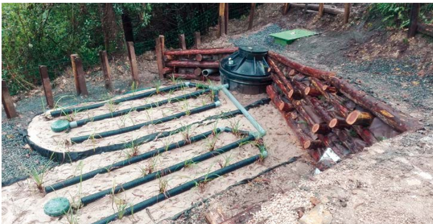
General appearance of the phyto-purification and mechanical-biological filtration system upon completion of the intervention.
